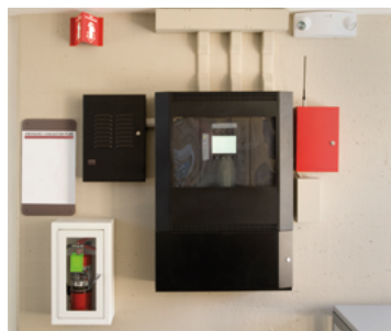
Security and fire alarm
